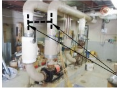
D2 CENTRAL MECHANICAL ROOM CHW BYPASS
