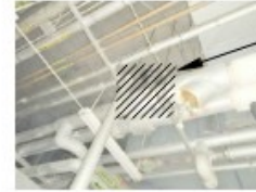
C1 AHU CHILLED WATER VALVE
