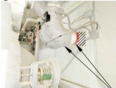
E1 WEST MECHANICAL ROOM HHW BLDG ENTRANCE
