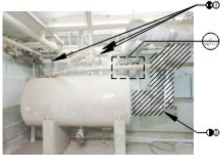
D1 WEST MECHANICAL ROOM EXISTING DHW HEAT EXCHANGER
