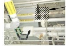
C2 AHU HEATING HOT WATER VALVE
