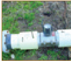
FIGURE VII.2 - Meter in pipe section mounted in a sprinkler system show portability
